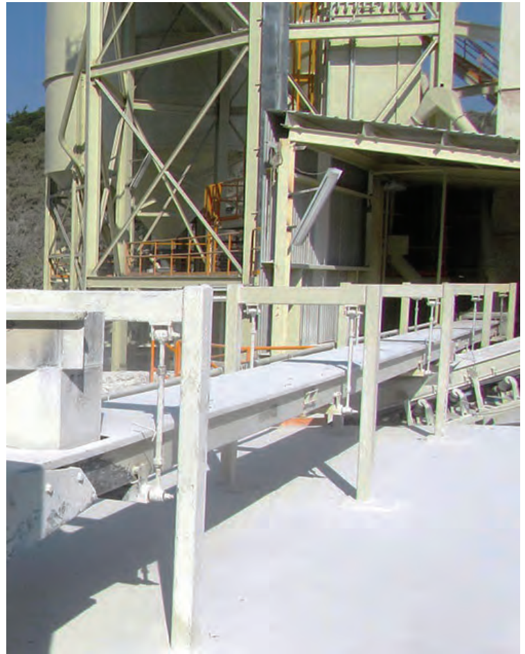
Horizontal motion conveyors moving quicklime.
