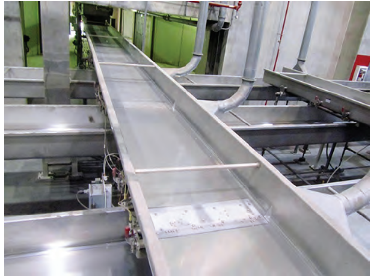
Horizontal motion conveyors replaced horizontal bucket elevators and reduced maintenance costs for a food manufacturer
